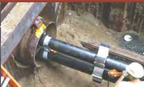
Ronkonkoma Hub Pump Station
