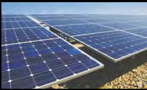
Smithtown Solar Photovoltaics
