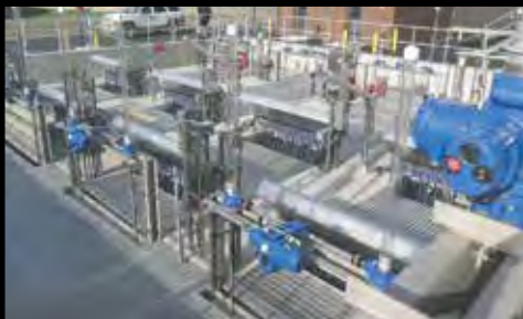
Bergen Point WWTP
